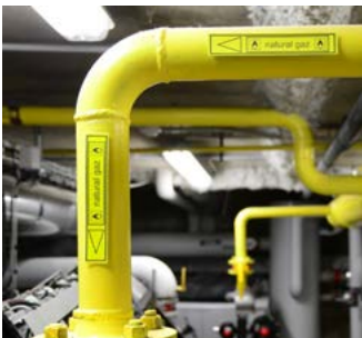
Pipes and valves identification
